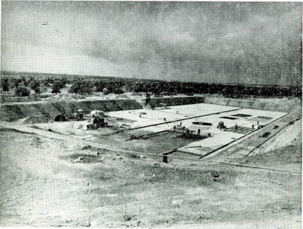
Concrete lined night storage reservoir 20,000 m 3 capacity belonging to Trakhoni extension of the Yermasoyia-Polemihia Project. It will be completed towards the end of 1978. The Trakhoni extension will finally irrigate 4,390 donums of citrus and vines. The whole Yermasoyia-Polemihia Project including Akrounda, Phinikaria, Yermasoyia and Polemihia Irrigation Divisions, Phasouri, Zakaki, Ayios Nikolaos and Trakhoni extensions will command an area of 16,000 donums permanent and annual crops. WDD photo A59-2.
