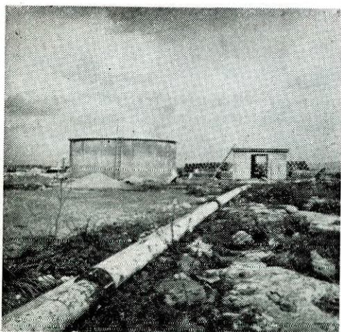
270 m3 capacity storage tank connected to Khirokitia-Famagusta pipeline near Phrenaros reservoir. A booster pump station (on the right) pumps water through an 8" dia steel pipeline to Paralimni and Ayia Napa villages to be used for their domestic water needs. WDD photo No. A72-6.
