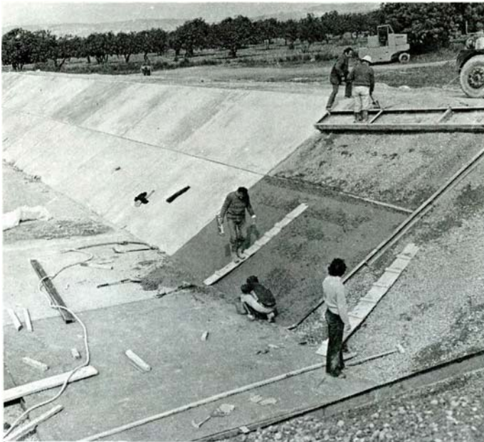
Irrigation network of Western area. Concrete lining of Kissonerga storage reservoir (4,000 m 3 ). WDD Photo D5-12 (11.2.82).
