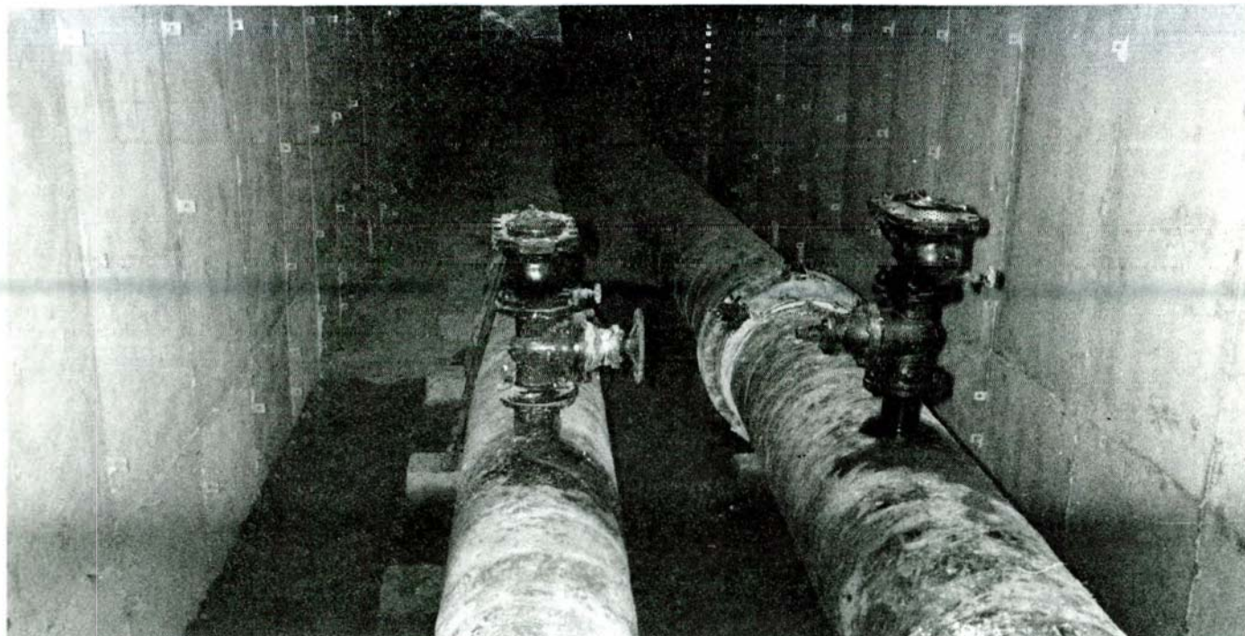
500 mm dia. Suction-Irrigation AC pipe (steel in culvert) with 550 mm dia steel Lefkara- Khirokitia pipeline within culvert under the new Nicosia/Limassol highway at Skarinou bridge. WDD Photo C 99-2 (14.1.82).
