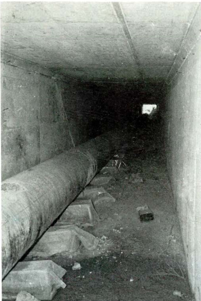
500 mm dia steel delivery main from Dhyptomamos Pumping Station to Stavrovouni/Kornos at culvert crossing under new Nicosia/Limassol highway at Kakoradja. WDD Photo C 97-7 (13.1.82).
