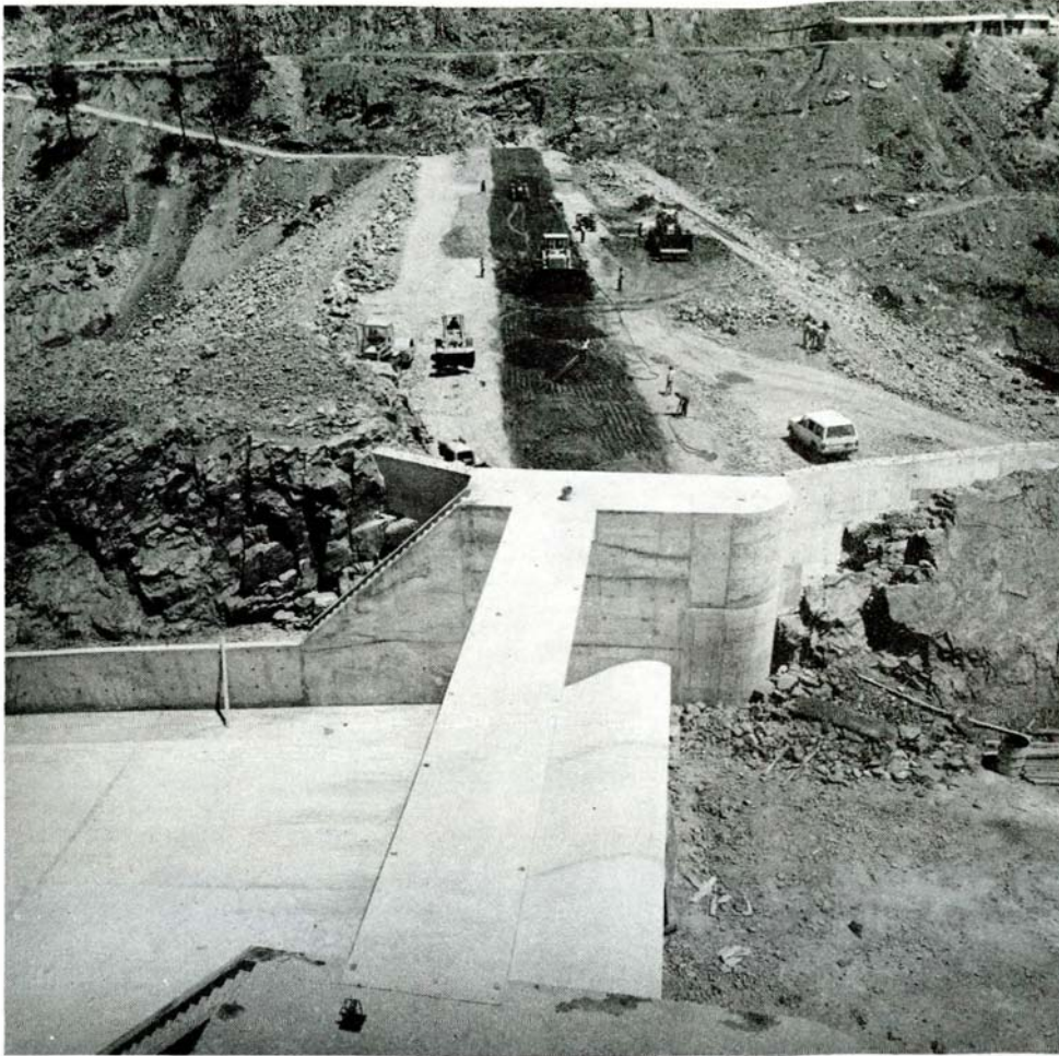
Xyliatos Dam under construction View from left abutment with concrete spillway in the foreground. WDD Photo D28-12 (5.7.82)
