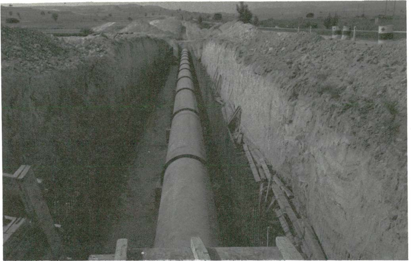
SCP - Main Conveyor. Culvert under the Larnaca-Kophinou Road. WDD Photo No. E19EN-24A (16.10.87).
