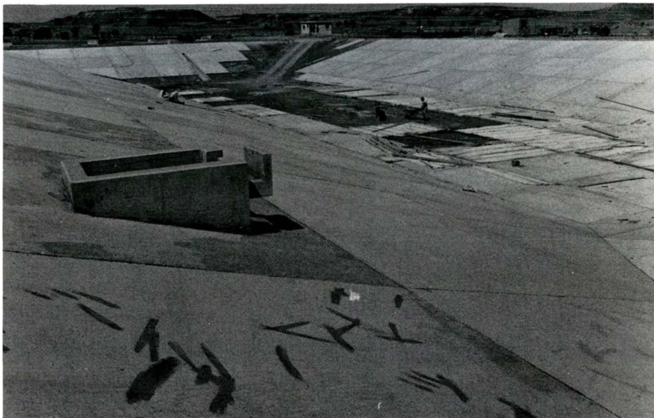
Ayios Sozomenos biological sewage treatment plant. Facultative aerated lagoon. WDD Photo No. D91EN-11 (10.6.87).
