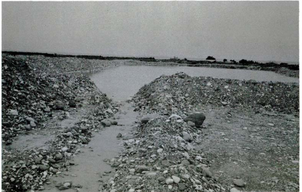
Fig. III-2 Kouris Delta recharge pond looking Downstream inflow in the Pond WDD Photo No. D62EN-17 (23.3.87)
