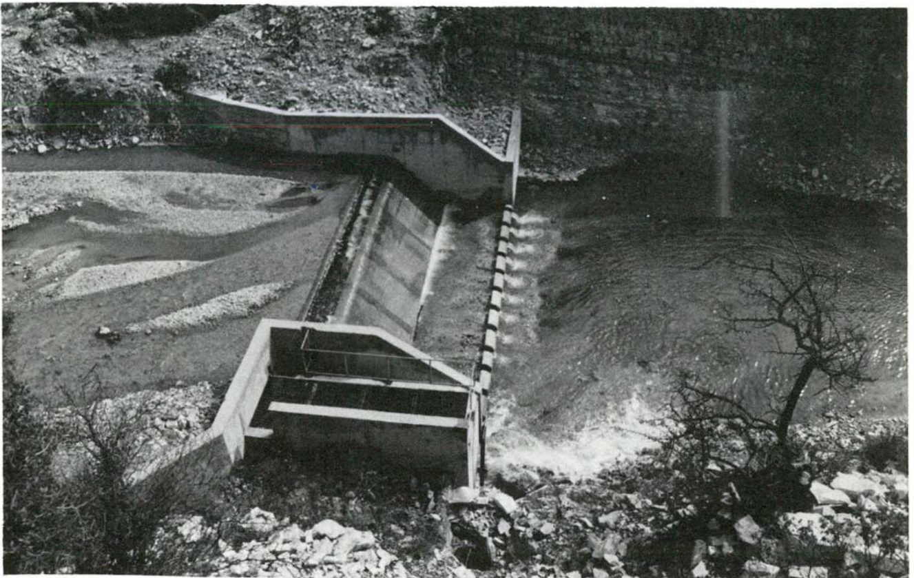
Evdhimou-Paramali irrigation scheme Diversion weir on Kryos river. WDD Photo No. E60EN-7.
