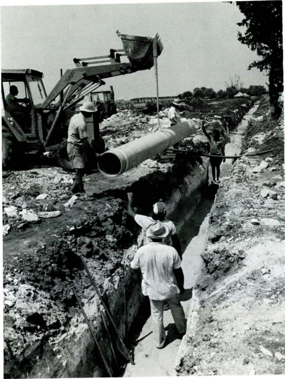
Kokkinokhoria Irrigation Area. Laying of 400 mm dia AC pipes. WDD Photo No. F28EN-5
