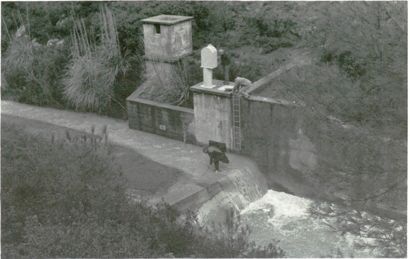
Mylou River flow gauging station at Kornos WDD Photo No. D58EN-15A (12.3.87)
