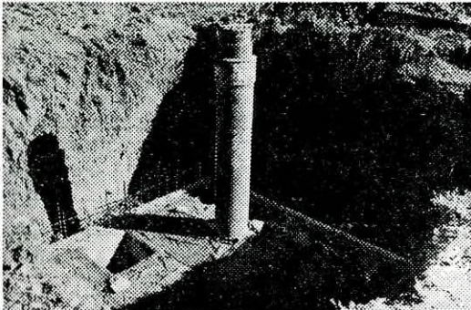
Construction of borehole well head. 24 such boreholes are included in the Paphos Irrigation Project.
