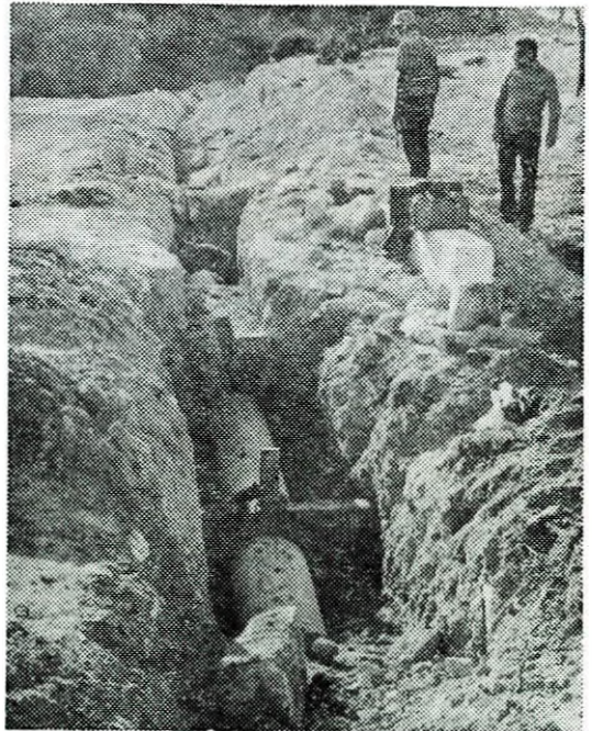
700 mm dia steel pumping main internally and externally coated being laid from Trakhoni pumping station to Trakhoni concrete lined reservoir, both belonging to the Yermasoyia-Polemihia Project.
