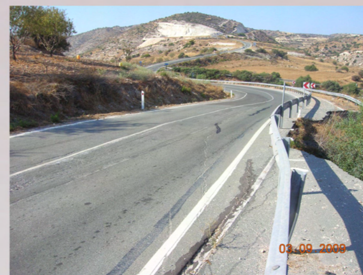
9. Fissures and settlements on public/central road of Ayias Varvaras-Pentalias caused by the adjacent landslide
