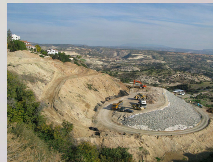
10. Stability measures-artificial slope construction-at the toe of the landslide (Pissouri village, photo 7 & 8)
