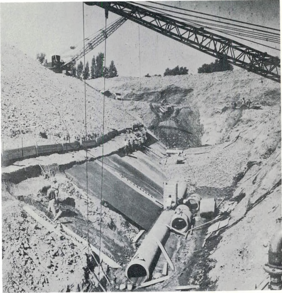
Infiltration gallery in the gravel deposits of Vasilikos river.
