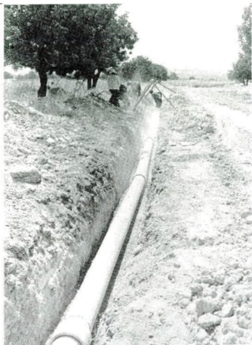
Installation of irrigation networks in Western Sectors. Pipelaying for distribution system of Kissonerga Sector in progress. WDD Photo C69-2 (6.8.81)
