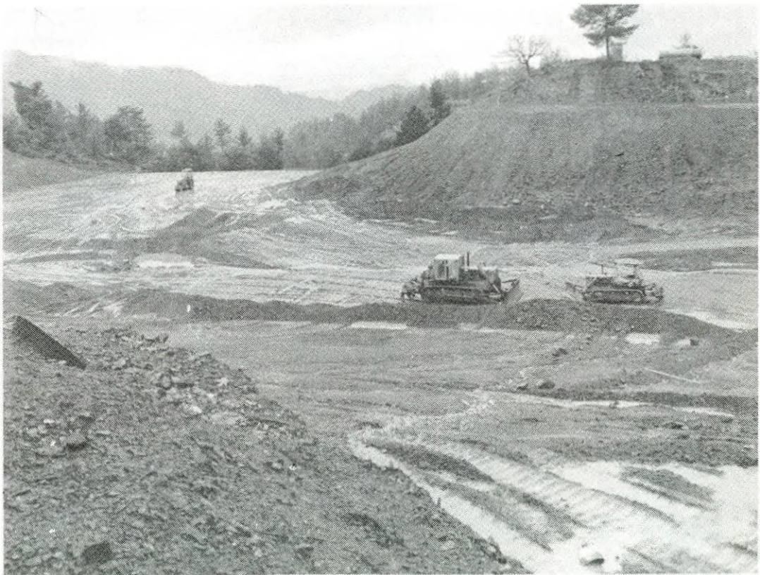
Kato Mylos offstream PVC lined pond under construction. This pond built within the Pitsilia Integrated Rural Development Project has a capacity of 104,000 m 3 of water for the irrigation of some 300 donums of land together with a borehole scheme, both belonging to Vatera Irrigation Division of Kato Mylos Village. WDD Photo C30-12 (6.2.81)
