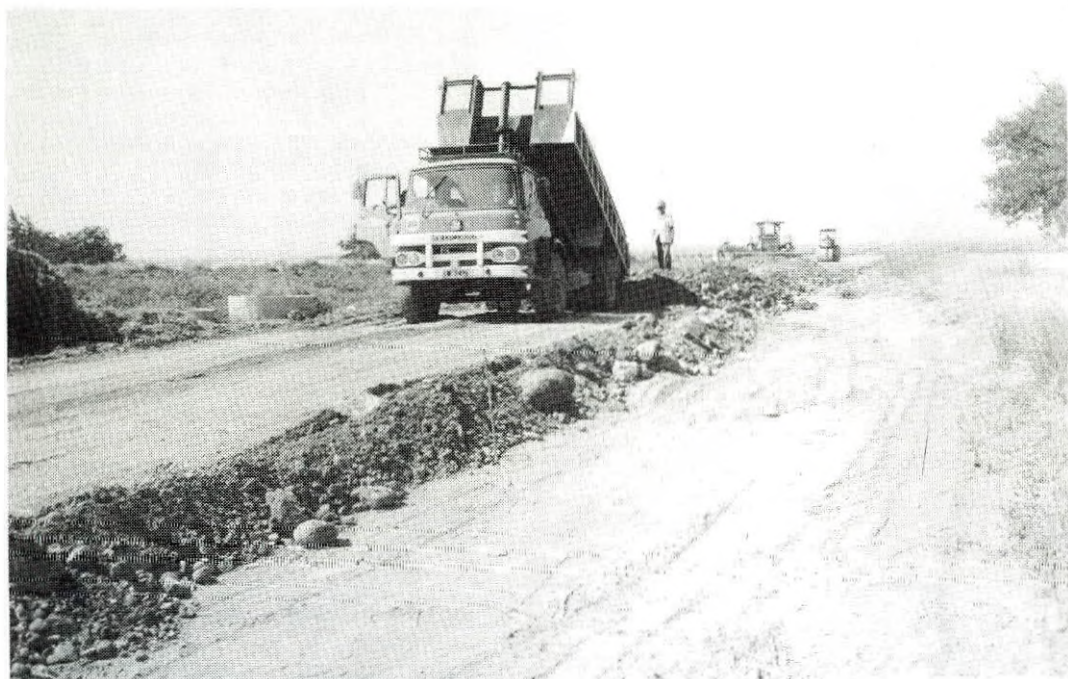
Placement of fill material (river gravels) on road embankment for construction of farm access roads in Eastern Sectors of Project. WDD Photo C59-11 (11.6.81)
