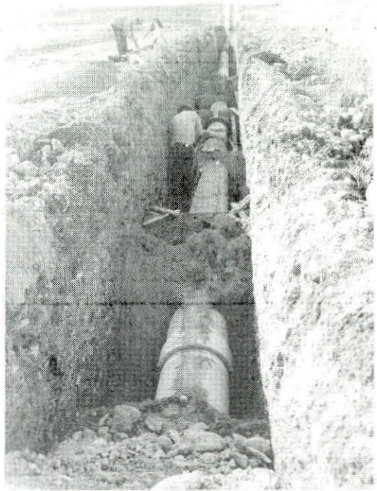
The laying of the 40 km long 600 and 500 mm steel and AC pipeline connecting the Khirokitia-Famagusta pipeline to Dhypotamos Pumping Station and from there to Stavrovouni Balancing Tank and on to Nicosia was substantially completed by the end of the year. The photograph shows a length of the 500 mm AC pipe being laid towards the Nicosia end of the pipeline. WDD Photo C43-11 (30.3.81)
