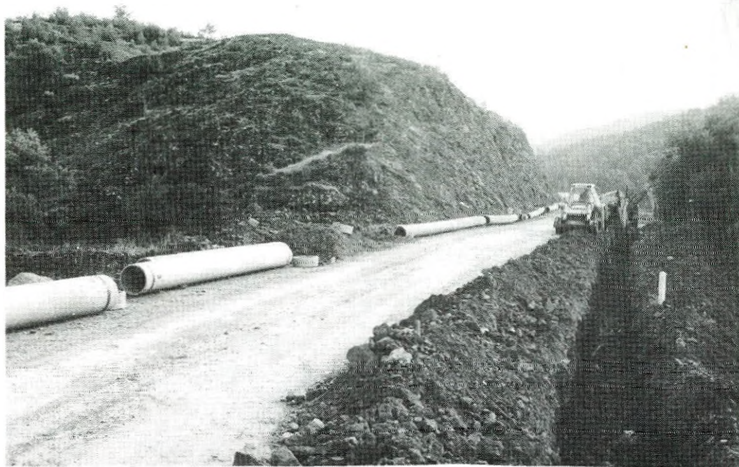
Water from Xyliatos Dam will gravitate to the area to be irrigated, some 2,300 donums, belonging to Xyliatos and Ayia Marina Villages. Work on the laying of the main conveyor pipeline commenced during the latter half of 1981. PIO Photo (11.1.82)
