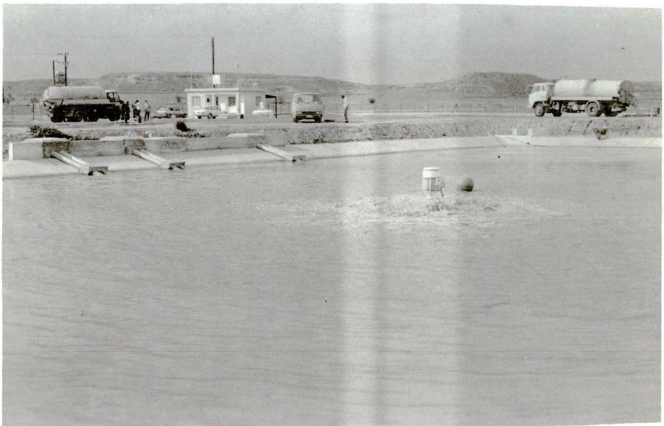
Aerated lagoon for pre-treatment of non-toxic waste of high BOD at Nicosia septage treatment plant (Ayios Sozomenos).
