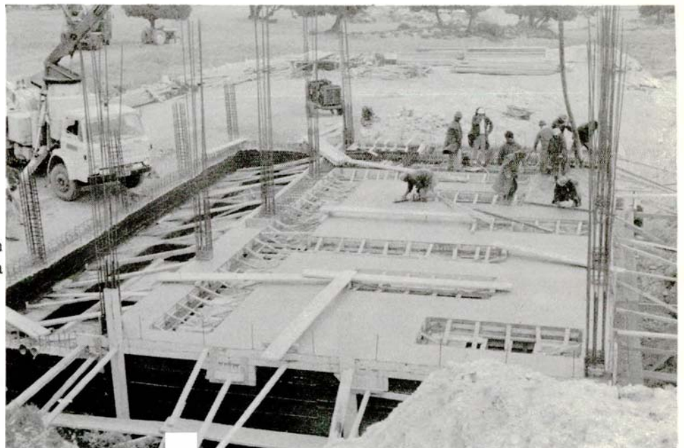
Kophinou pumping station under construction on Khirokitia-Phrenaros pipeline. Booster pumps will be installed to increase the water capacity of this important pipeline which feeds Larnaca, Famagusta several villages and the tourist industry in the homonymous districts. WDD photo F7EN-23A. Taken on 27.5.88
