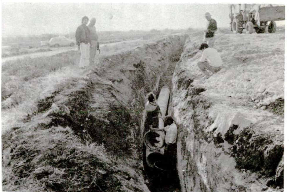
SCP Contract C7 (Force account). Installation of 400 mm AC pipe of irrigation bock X of Kokkinokhoria Irrigation system. WDD photo F56EN-7. Taken on 8.12.88
