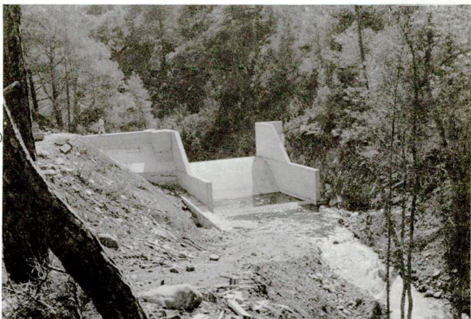
Diversion weir structure on Magounda river. Surplus winter flows (after the filling of Argaka dam downstream) will be diverted to Evretou dam. WDD photo E79EN-18. Taken on 15.3.88.
