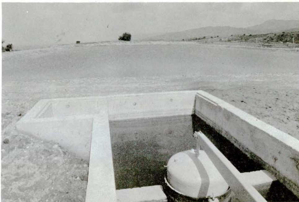
KIP irrigation distribution system storage pond with its inlet break pressure tank. WDD photo E78EN-11. Taken on 15.3.88.
