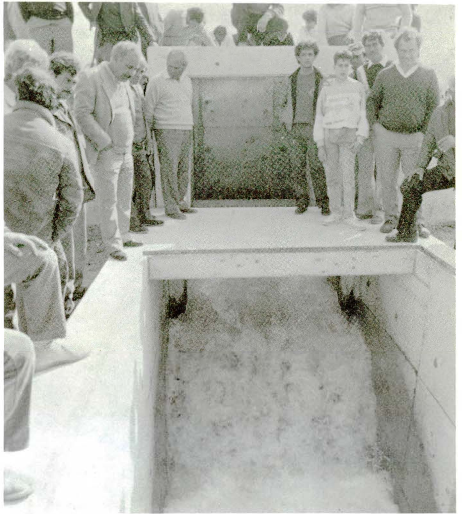
The first flow of water from Kouris dam through the 110 km long, 1400-800 mm dia DI pipeline from Kouris to Akhna dam reservoir. WDD photo E58EN-9. Taken on 9.2.88.
