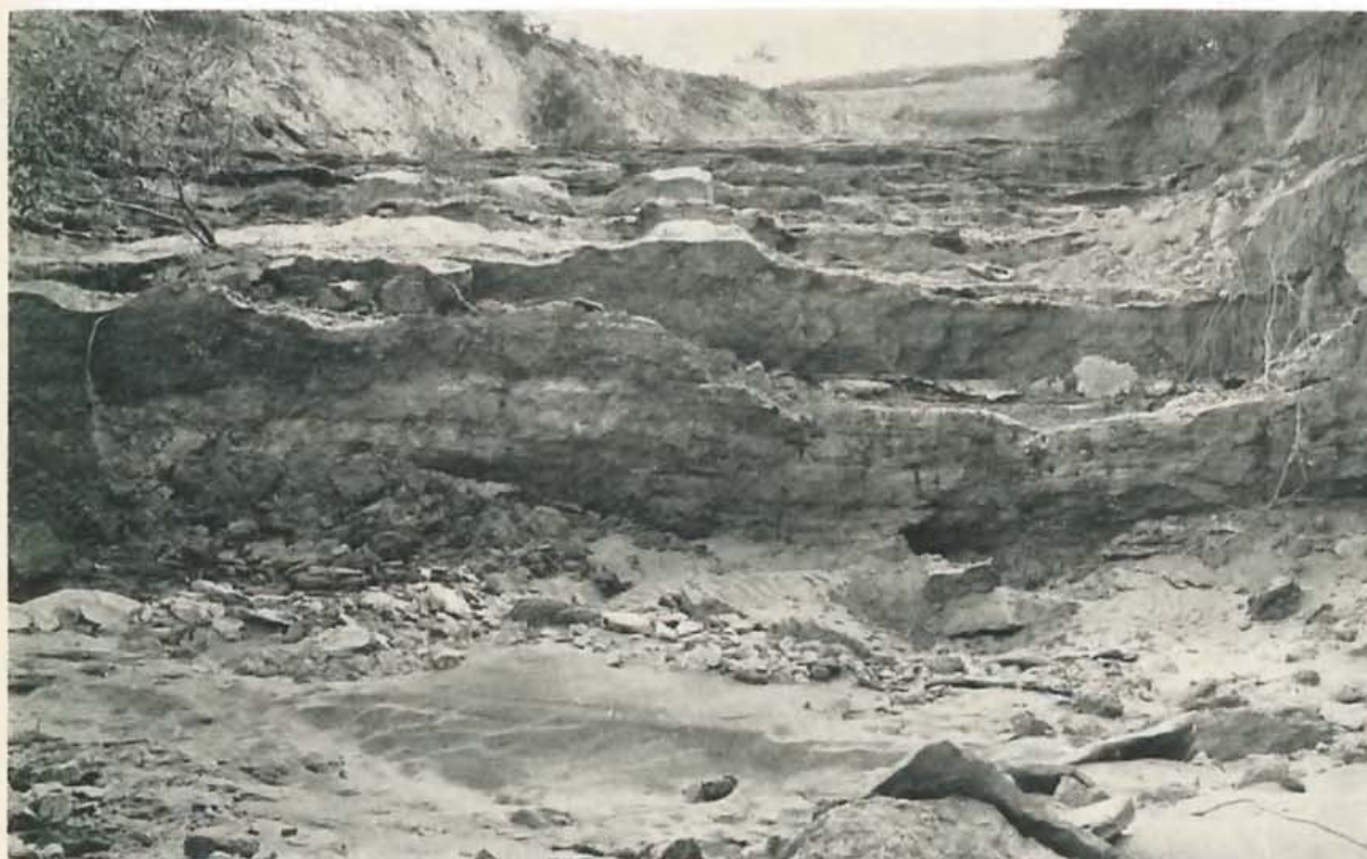
Erosion of unlined spillway.
