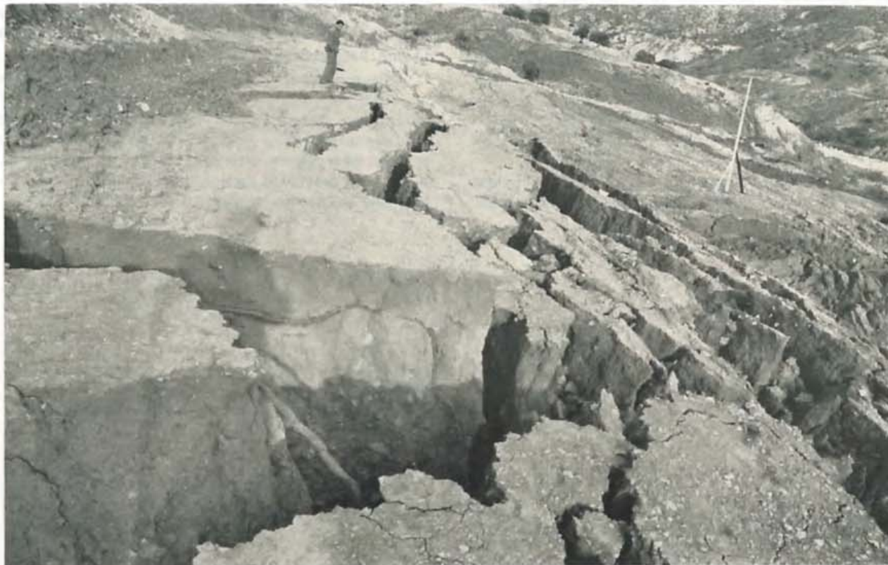
Reservoir slide area on the right abutment.
