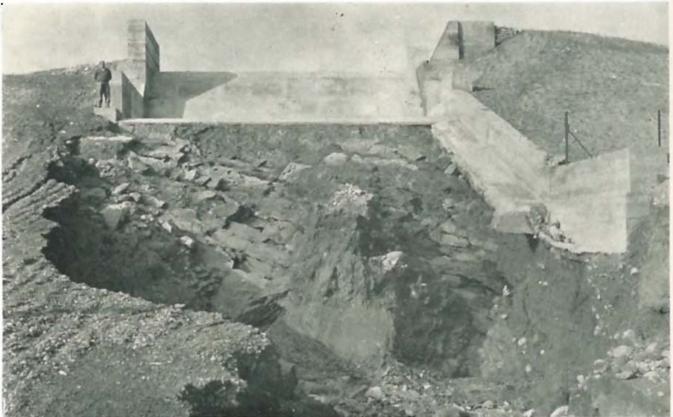
Erosion of spillway unlined channel.
