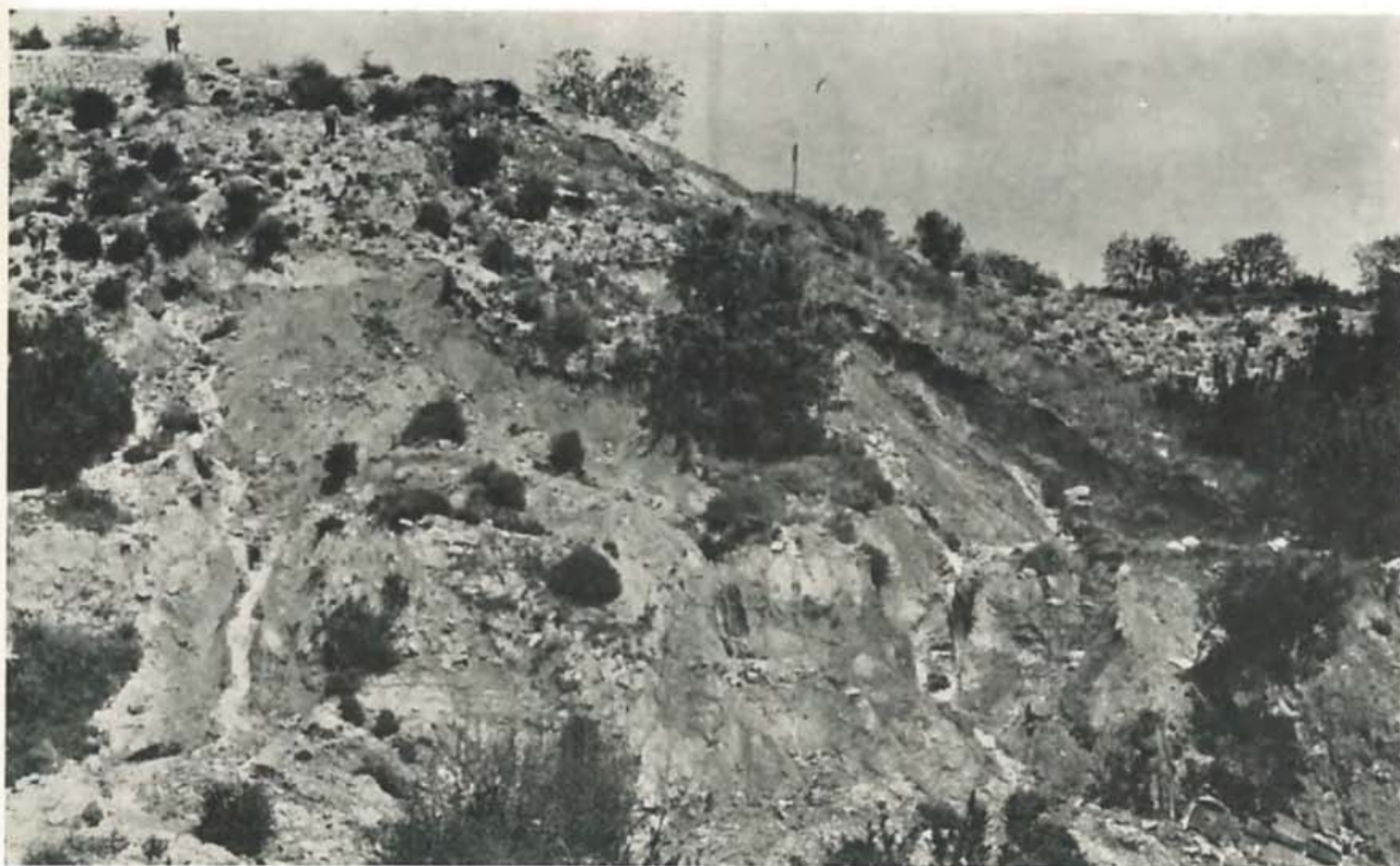
Extensive seepage with landsliding on the East abutment.
