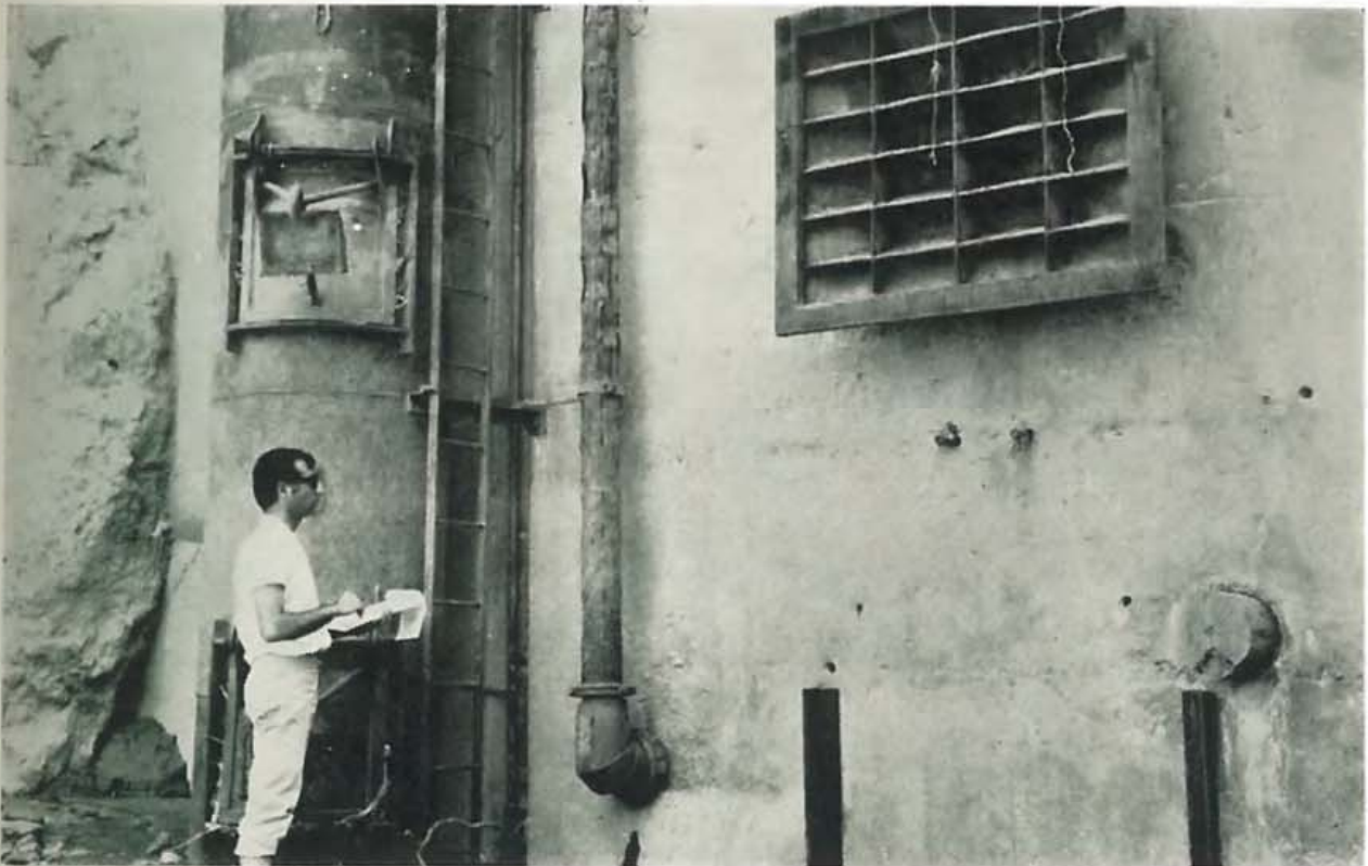
Trimiklini dam. — Desilting pipe with trap gates.
