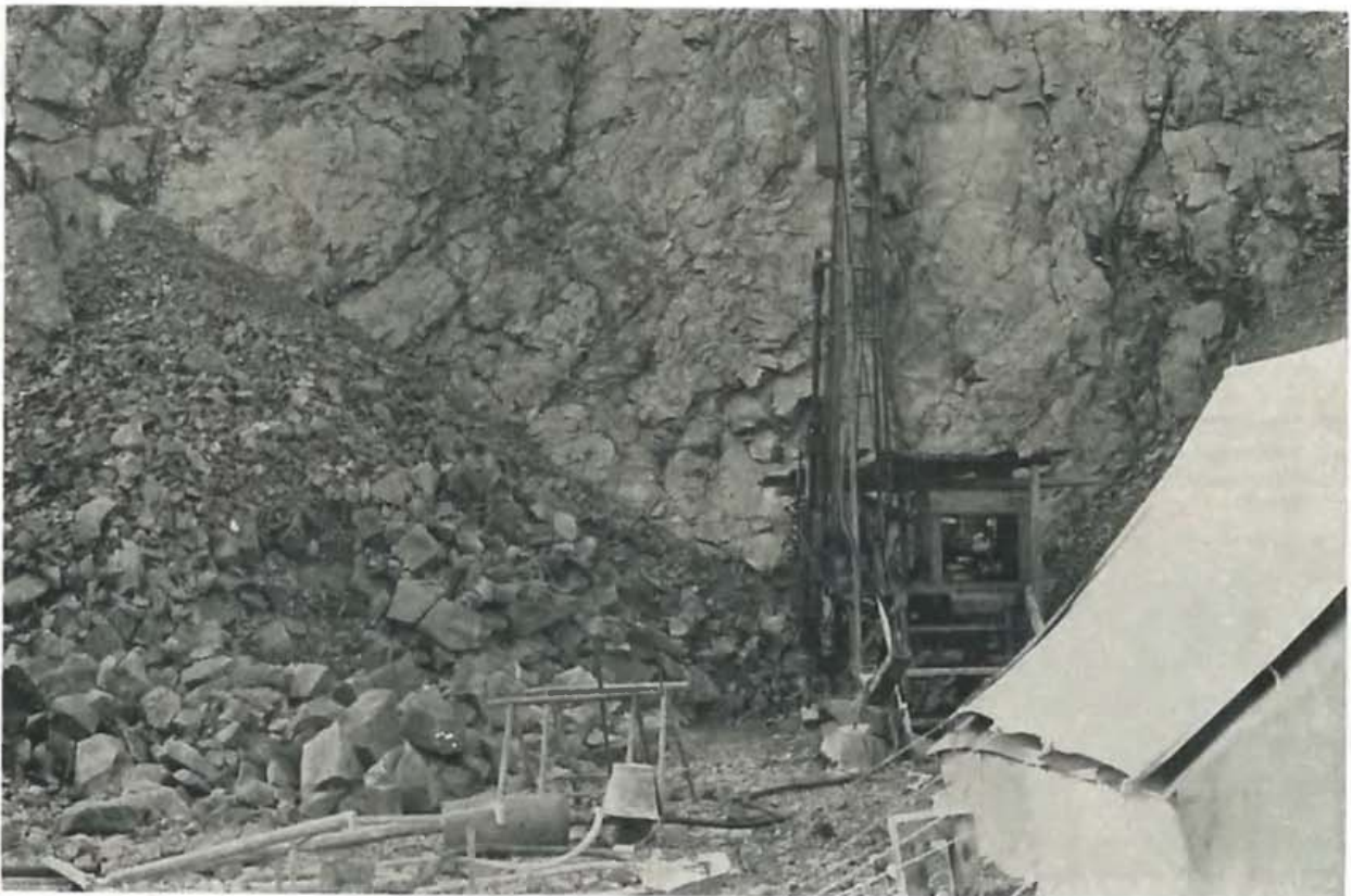
Drilling and grouting on the West abutment. Weathered and sheeted diabase rock can be seen.
